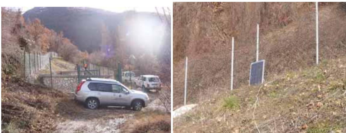
Figure 6.5 Station 09 located outside Norcia. The station was equipped with a solar panel due to the lack of nearby power supply.
